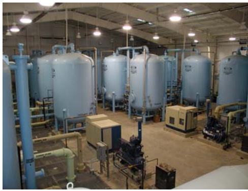
Unique Tertiary Carbon Filtration System
