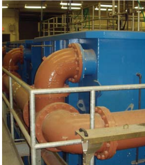
HRC designed a tertiary treatment system never before used in a wastewater treatment application in Michigan, using Enhanced High Rate Clarifiers, commercially named Actiflo®.
