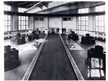
Picture No. 2—PUMPING STATION, SHOWING SIX MAIN PUMP MOTORS.
