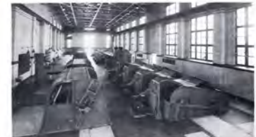
Picture No. 3—RACK & GRIT BUILDING WITH BAR RACKS ON LEFT AND GRIT COLLECTORS ON RIGHT.
